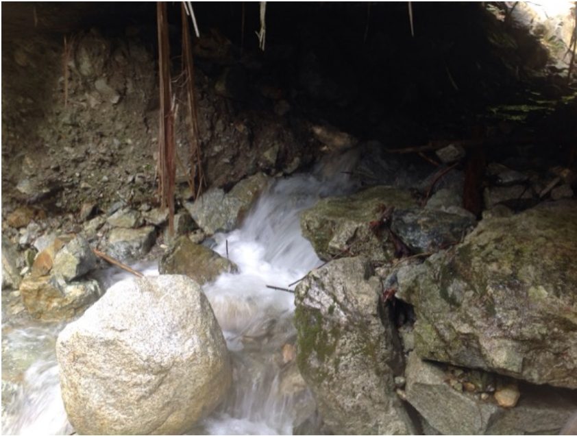
stream erosion is leading to abutment erosion
