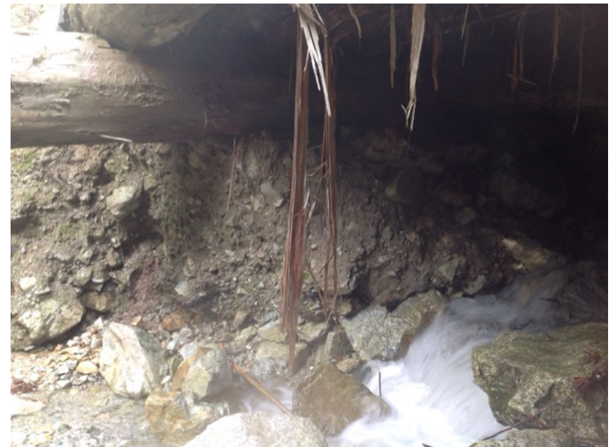
right bank abutment erosion
