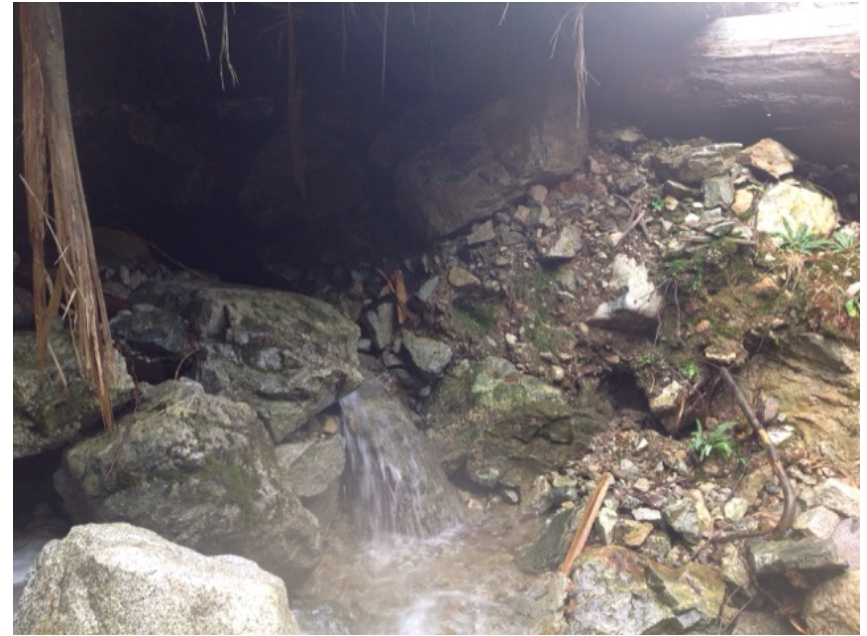
stream erosion leading to abutment erosion
